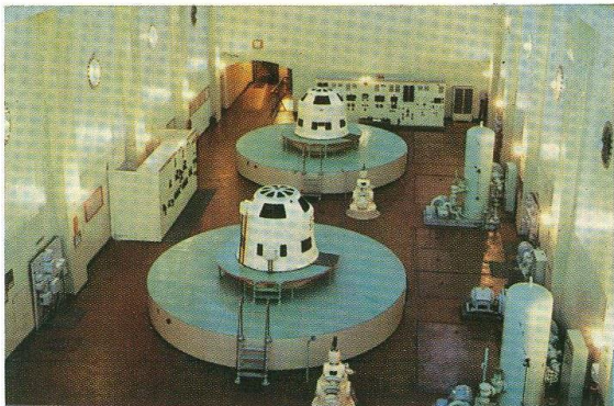
Sevan Hydroelectric Power Station. Underground Turbine House
